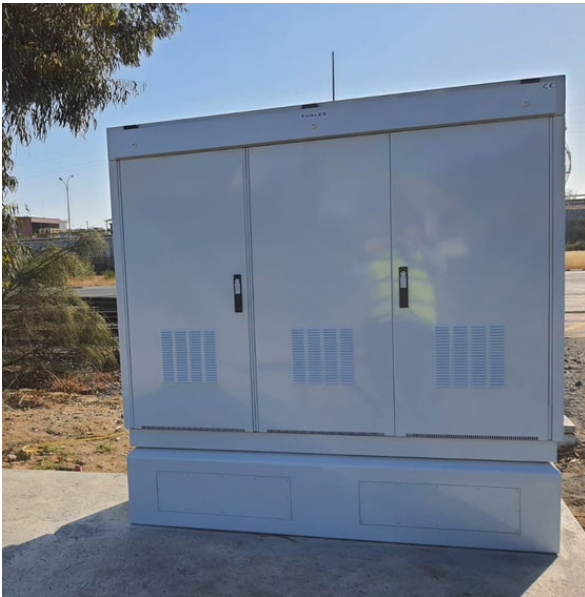
Figure 2-3 Typical Object Controller Cabinet (OBJ)
